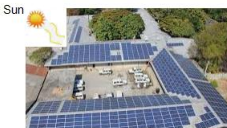
Fig. 5: Solar panels on hospital roofs.
